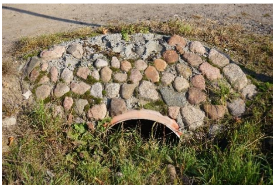
Image 3. A blocked culvert no longer allowing water to flow through it.
